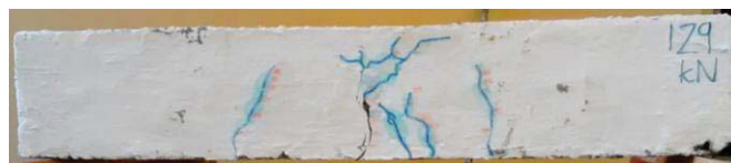
Fig. 13 Crack pattern of MKHSFB-F
